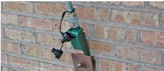
The Simplex S2000A spreader was used to remove this rusted anchor plate from a brick wall for mortar patching to begin. ▼
